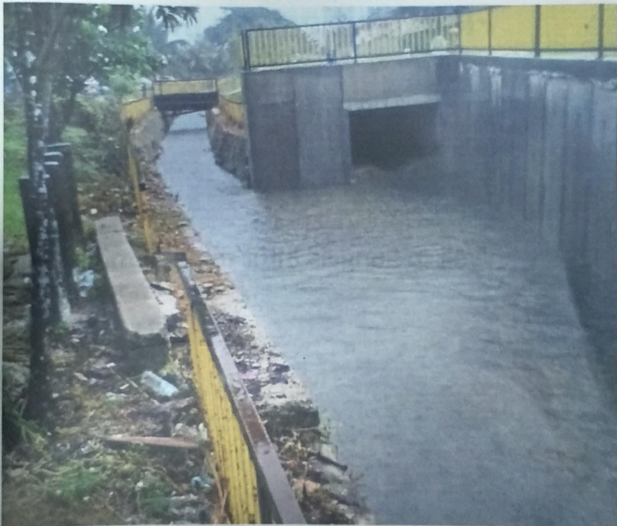
High and dry: The tunnel (at right) built to channel water to the underground flood retention pond in Taman Nirwana in Ampang Jaya, Selangor, is too high and ineffective to handle the volume during heavy rain.
